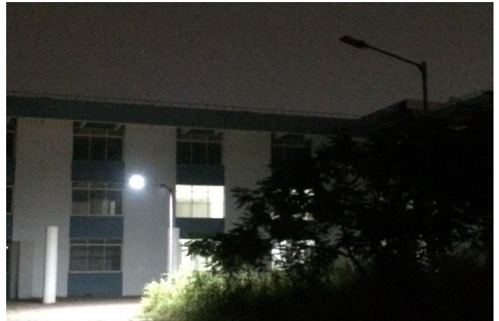
Image showing an audit location with non functional streetlight.
